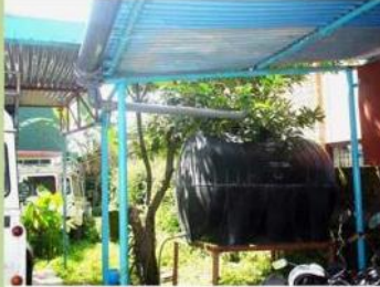
RWH technology installed at NEWAH HQ
